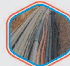
Underground Electricity Fitting
